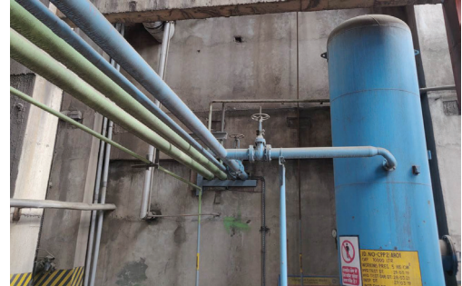
Figure 31: Existing compressed air piping
